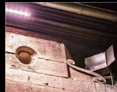
These Parade S-RGBW-20 spotlights were fixed below the eaves.
