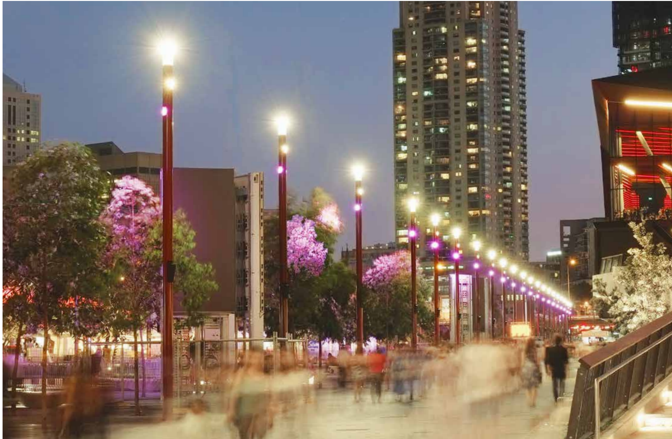
A total of 30 specifically modified CITY ELEMENTS were installed along the Darling Harbor Boulevard. All lighting modules are linked to a DMX controller.
